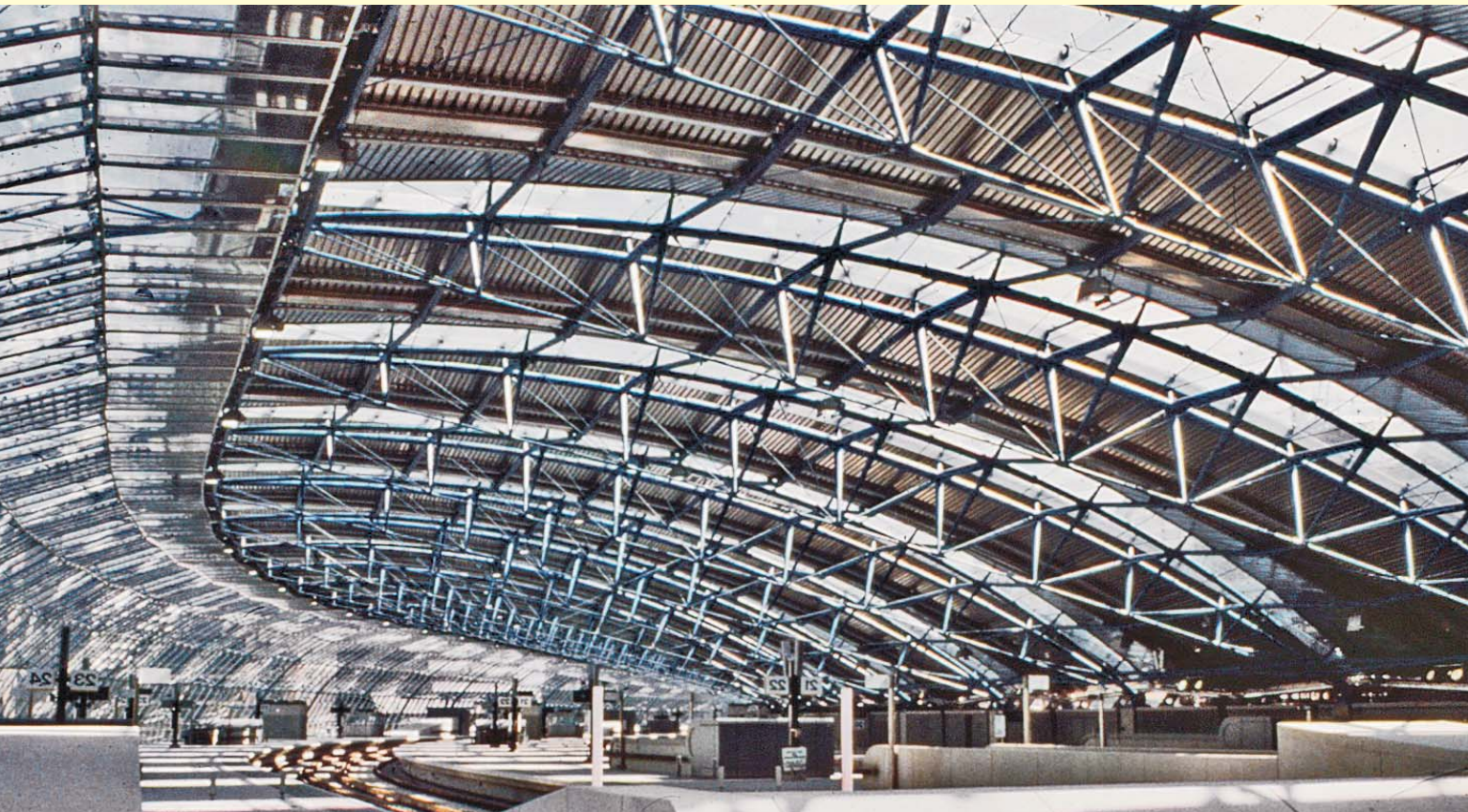
The designers of London's Waterloo Train Station used Type 316 stainless steel for roof structural supports and panels, slip resistant flooring and stair treads, ticket booths exteriors, railings and other items. (Figure 2) Photo courtesy Nickel Institute
