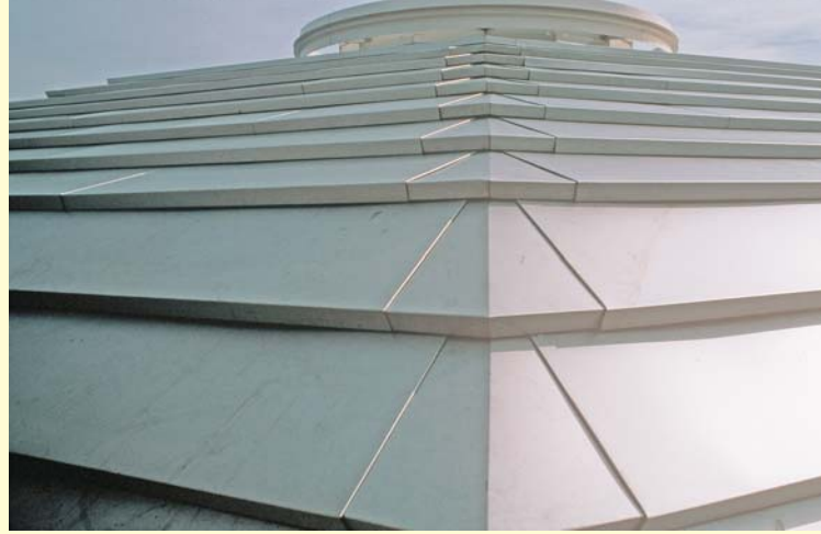
Type 304 with a custom dull finish was used for the Bermuda style roof on Ronald Reagan Washington National Airport. It was also used for interior ticket counters, elevators, signage and other applications. (Figure 3a) Photo courtesy Overly Manufacturing Co.,
